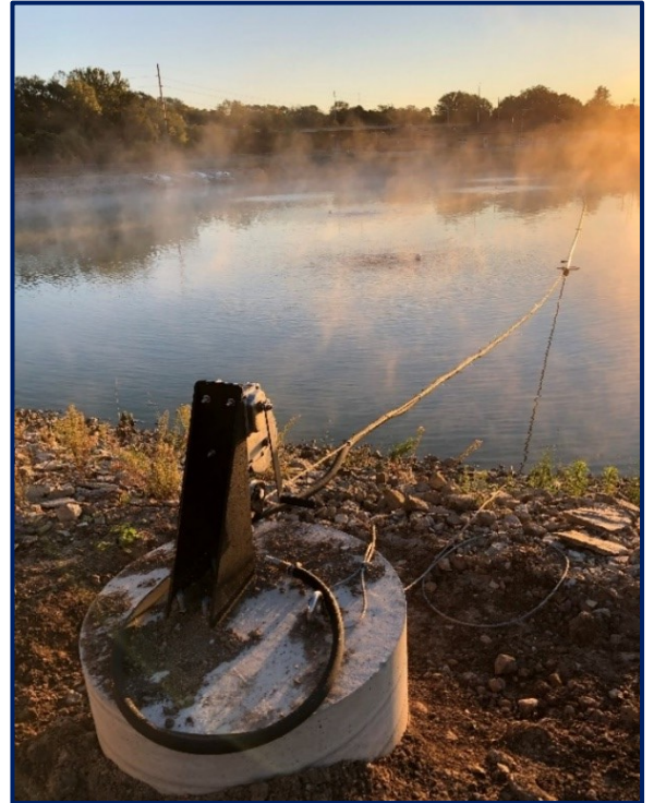
S.S. wire rope and hand crank anchor each floating header to shore
