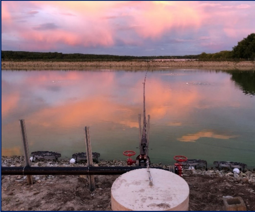
Floating HDPE connects to HDPE feeder pipe supported by galvanized posts
