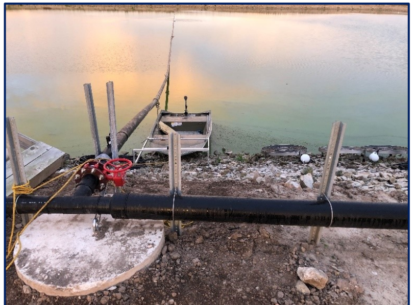
Feeder pipe connects to a tee and floating header pipe with saddles for each diffuser
