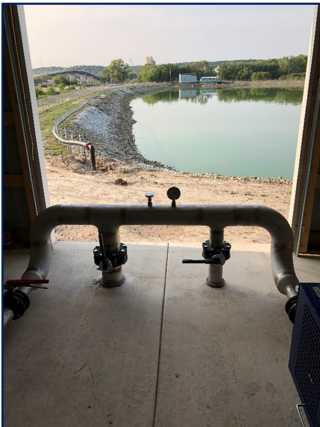
Blowers connect to underground metal piping to dissipate heat
